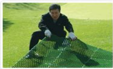
7 The mats should be pulled in every directions to make them flat to not be lifted.
